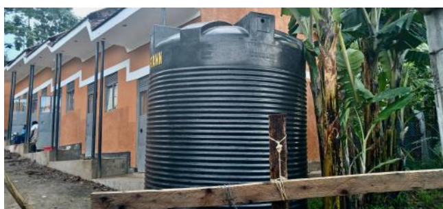
Rain Water Harvesting in Staff Compound
